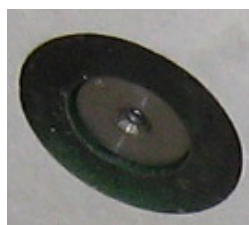
Wrong fixed on the formwork
