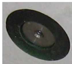
Wrong fixed on the formwork
