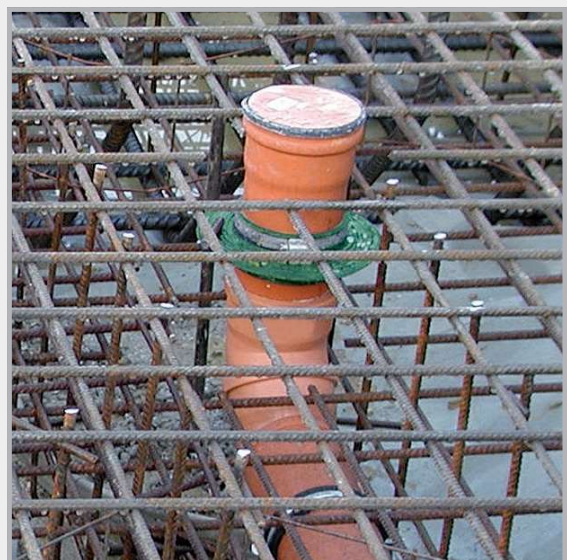
The RONDO, shortly before placement of concrete. The drainpipes are securely and permanently sealed against rising moisture.
