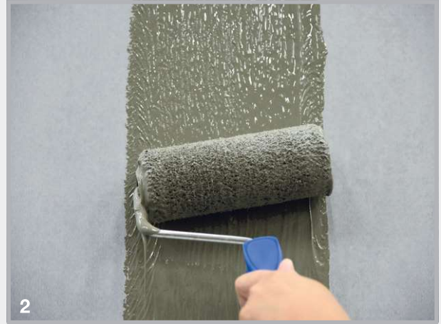
2 Apply the first coating layer. Layer thickness: approximately 1.2 mm Usage: approximately 0.6 kg per metre/joint
