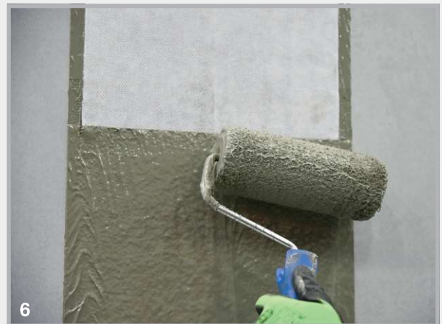
6 Apply the second coating layer. Layer thickness: approximately 1.2 mm Usage: approximately 0.6 kg per metre/joint The edge area of the non-woven must be completely covered.
